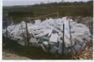
Big-tilt cast-in-place concrete forms allowed them to build the building's unique structure. These materials are shown on-site ready to be recycled.
