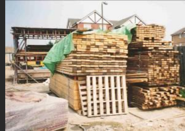
Reclaimed timber -from local demolition site -re-cut and used for internal stud work
