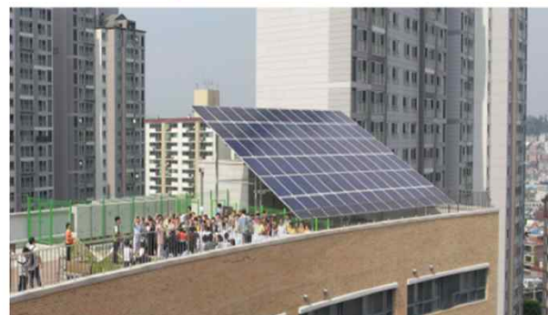
[ Sangaksan High School, 20kW, Completion '13.6.14 ]
