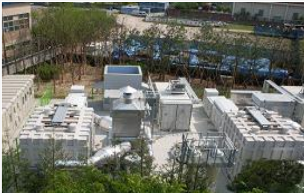
[ SH District Energy Site Sanggye area: 2.8MW ]
